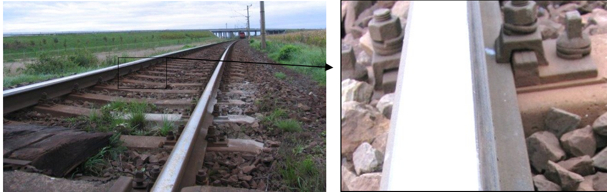
Fig. 2 The track irregularity and the wearing on the left side rail
