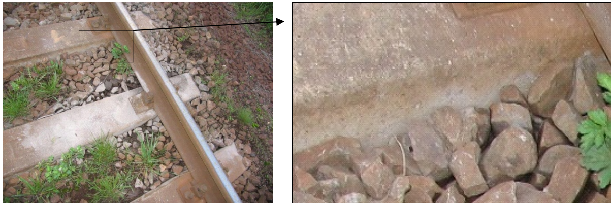
Fig. 3 The track irregularity (sinking) at right side rail, the sleepers and the ballast
