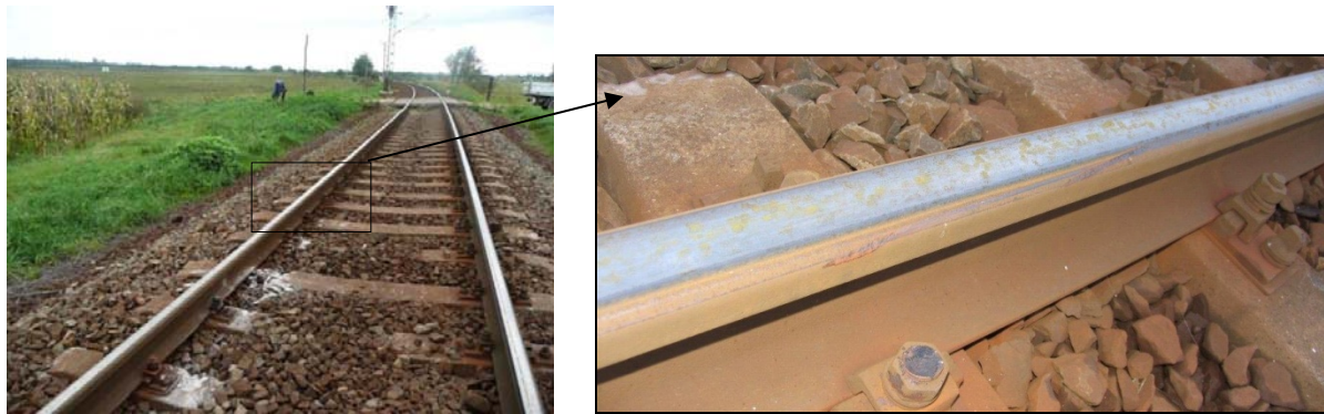
Fig. 6 The trace of derailment on the sleepers and on the inner side of the right rail
